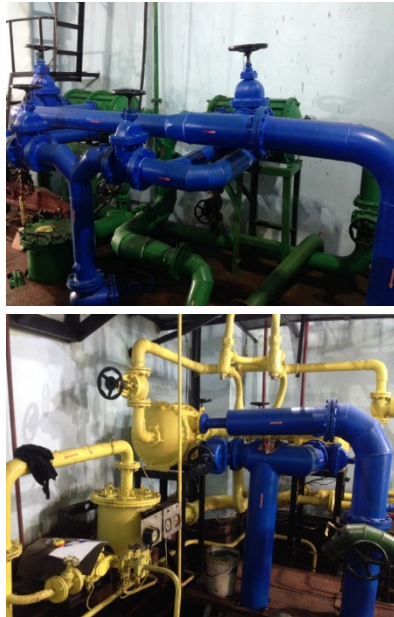
Fig. 7. Original cooling fluid and lubricating oil piping system on the M500 engine test bench
