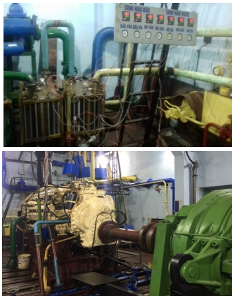
Fig. 8. Installation and testing of a cooling plate on the M500 engine test bench
