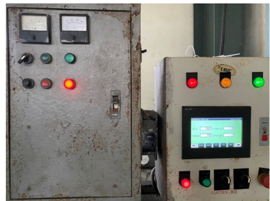
(c) Power supply unit and PLC controller
